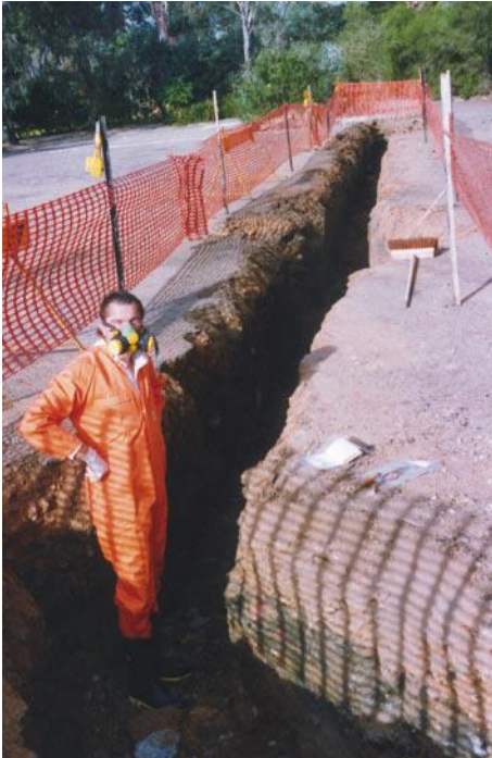
Philip Mulvey, Principal of Environmental & Earth Sciences Pty Ltd, carries out an inspection following a burst gas line.
